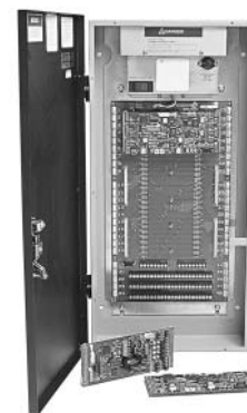
PRC100SCC Control Cabinet with Application Specific Controllers
